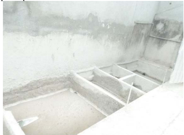
Fig. 2 Decanting system for wastewater of CA2.
