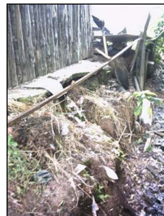
Fig. 11 Fluvial erosion of the margins.
